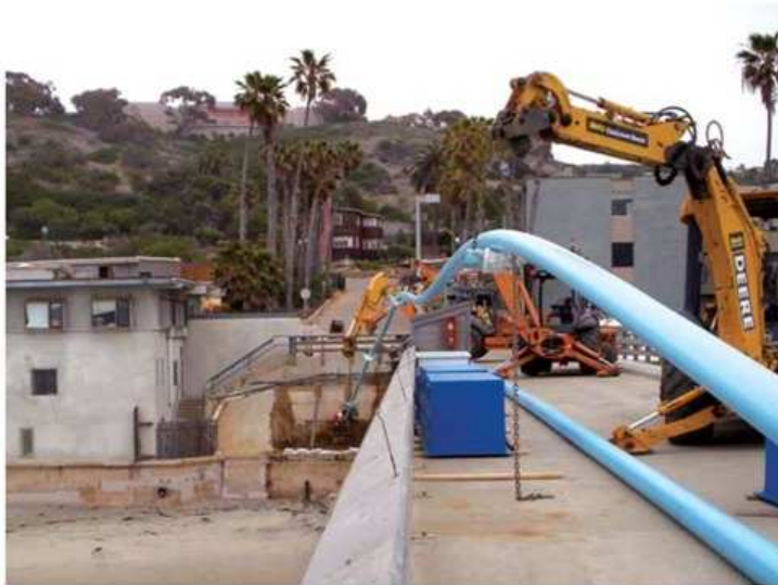
The project involved the fusing and installation of 3,000 feet of 8-inch Fusible C-900 pipe for the new seawater return system.
