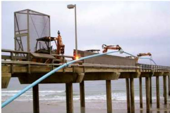
The specially made PVC pipe is fastened into place along the Scripps Pier as one long piece.
