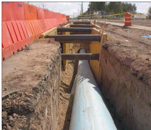
Project officials say this project marked the first time that 24-in. Fusible PVC was used on an HDD project of this size.
