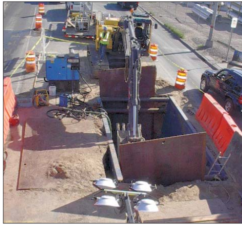
The project took place on an extremely busy section of highway at the Texas-Mexico border.
