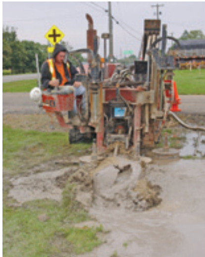
A Ditch Witch JT2720 is used on the directional drilled portion of the Riga Township water main project.
