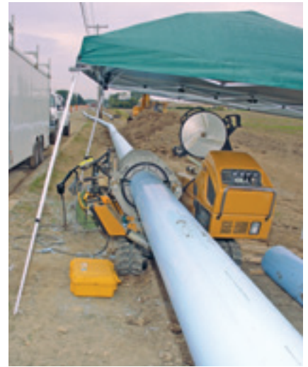
12-inch C-900 polyvinyl chloride water main is fused together for the Riga Township project.
