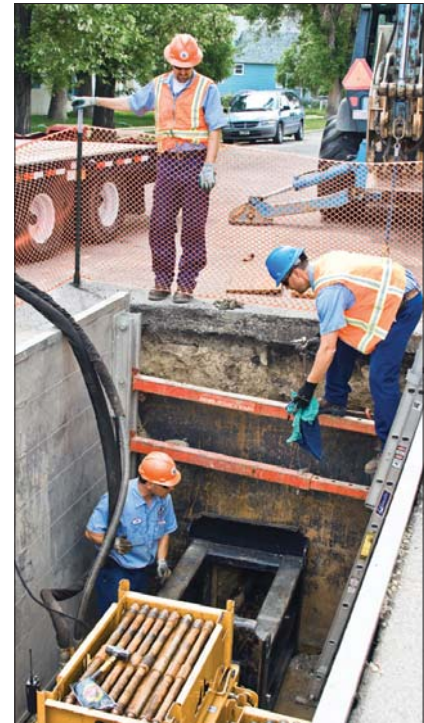
J.R. Fox (in excavation) realigns the HammerHead pulling unit while Scott Haynes (right) and Ryan Skillestad assist.
