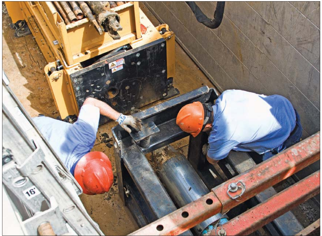
Senior equipment operator J.R. Fox (right) and maintenance worker/equipment operator Jim Burchell operate the HammerHead 100-ton hydraulic pulling unit.
