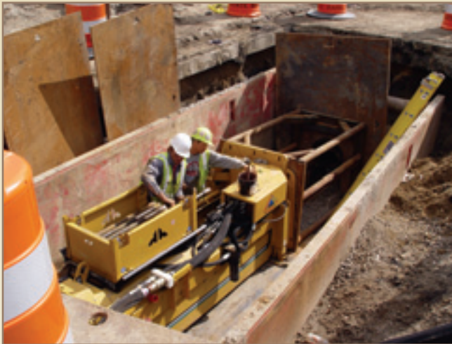
A Vermeer HammerHead HB 125, 125-ton static pipe bursting machine installs Underground Solution Inc.'s polyvinyl chloride pipe on the project.
