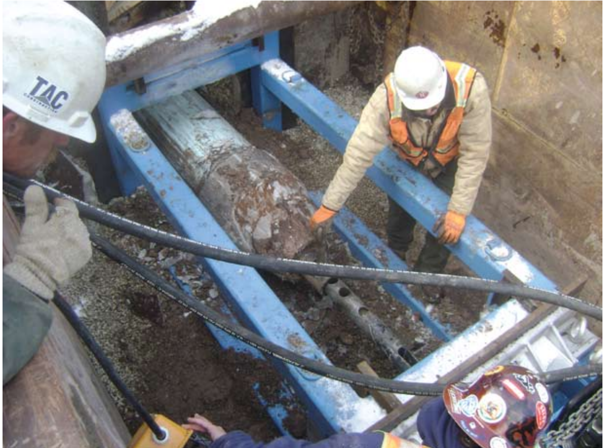
It took only four hours for the static bursting machine to burst over 800 linear feet of asbestos-cement pipe and pull in the replacement.
