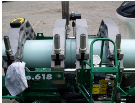
The joined pipe segments are held under pressure until the newly-formed joint cools sufficiently to ensure strength.
