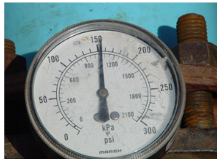
The taps were pressure tested to 150 psi for a period of one hour with no leakage. Both the dry and wet taps were successfully pressure tested.
