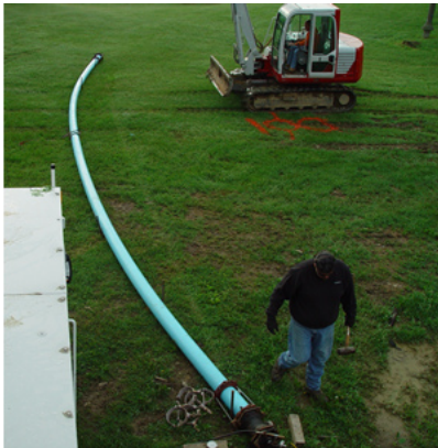
A 60-foot length of 6" DR18 Fusible C-900® with two fused joints was positioned to the recommended radius of 144 feet. Three quarter-inch saddles and corporations were used.
