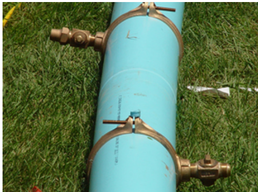
Taps were performed and corporation stops were installed at 12 o'clock, 9 o'clock, and 3 o'clock orientations. They were also located about 18 inches from fused joints.
